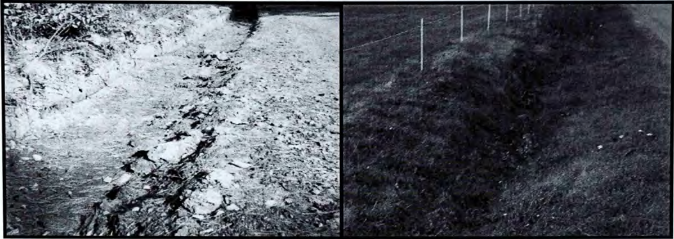
Figure 41. The photograph at the left is an example of a bad ditch because it is square in shape and is composed of bare soil. The photograph at the right is an example of a good ditch because it is parabolic in shape and is vegetated.
