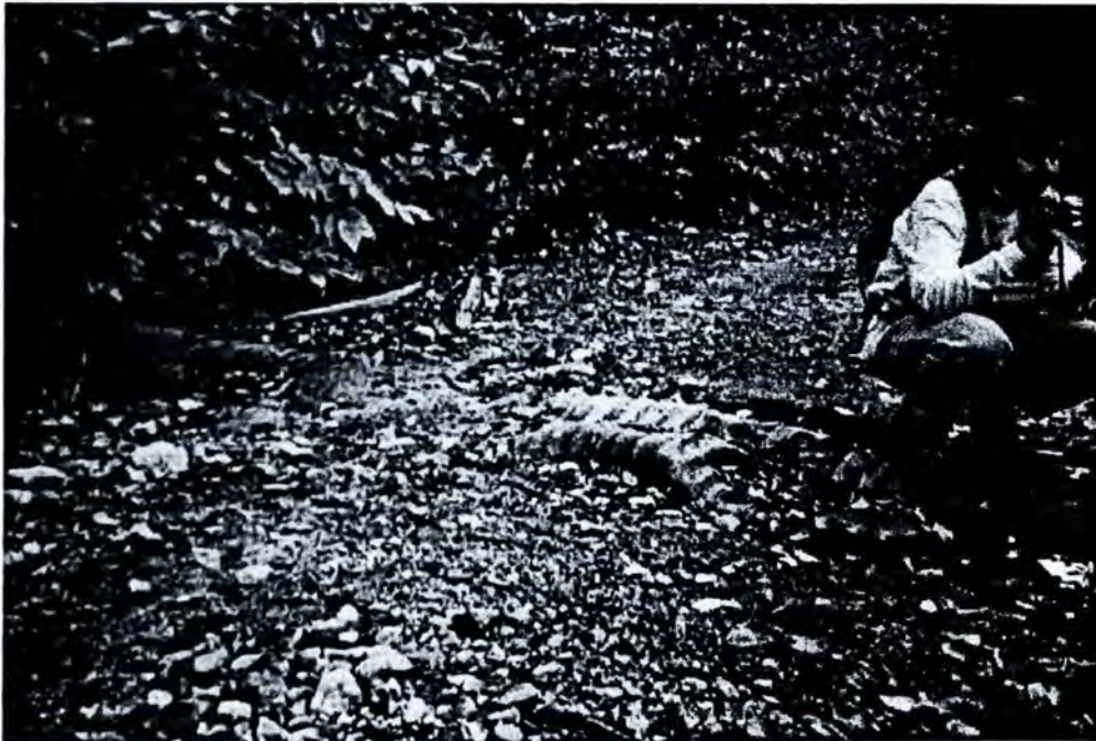
Figure 45. A poorly placed culvert in a dirt road which has not been properly maintained. This culvert should have been placed further below the road surface.
