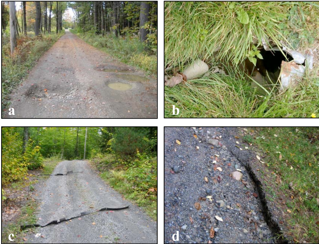
Figure 23. Examples of road problems in the Salmon/McGrath watershed. (a) A road with deep potholes. The road should be regraded to eliminate the potholes and improve crowning. (b) A culvert that is crushed and overtaken by grass. The culvert is also rusting. This culvert needs maintenance or replacement. (c) Rubber bars in disrepair. These rubber bars will not divert water properly and should be replaced. (d) A road with extensive erosion. Structures should be added to improve the removal of runoff from the road surface, such as rubber bars or ditches.
