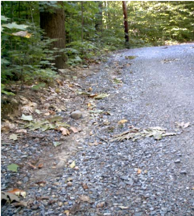
Figure 23. Example of a poor quality road within the Long Pond South watershed. Photo shows a road in need of ditches to divert runoff. As runoff is trapped by the berm on the left, the water erodes channels and causes debris to build-up.
