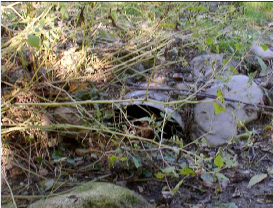
Figure 22. Good (top) and bad (bottom) culverts. The top culvert is large enough to allow proper water flow. The bottom culvert exhibits blockage by debris and a cluttered path for water flow. Photo credit: LMNO Engineering 2007.
