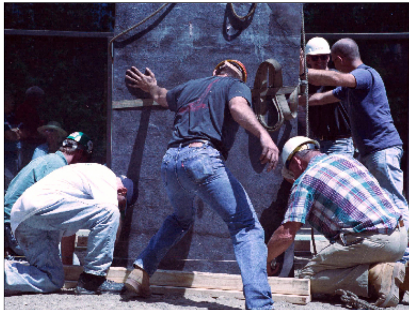
An installation crew, with sculptor Richard Serra kneeling at left, positions one of three 30-ton steel blocks that compose Serra's sculpture 4-5-6.
