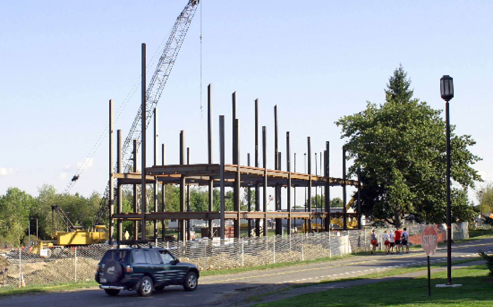
The framework of the new Diamond Building, a major academic initiative that will offer new opportunities in social sciences and interdisciplinary studies. The Diamond Building is part of a dramatic expansion of facilities included in the Strategic Plan for Colby, launched in 2002.
