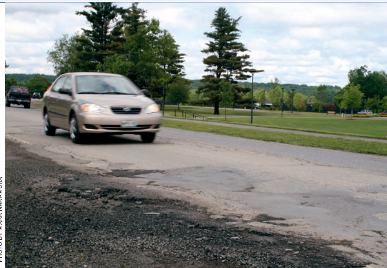
Increased pedestrian traffic and deteriorating road conditions led Colby to take over a mile of Mayflower Hill Drive. Plans call for reconstruction of the road, including the portion shown here, across from the Diamond Building.
