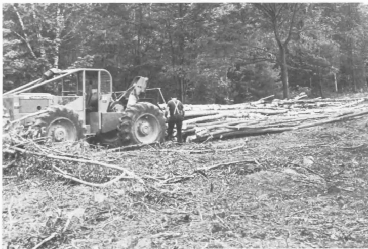
Preparing the site for the new 100-bed dormitory involved clearing and thinning over two acres of wooded land this summer. Logger Carroll Kinney says the work keeps him young. To be located on the hillside south of Lorimer Chapel, the two-story structure will incorporate significant energy conservation measures. Occupancy of the college's forty-second building is scheduled for September 1981. Architects are Philip M. Chu Associates of Chappaqua, N. Y.
